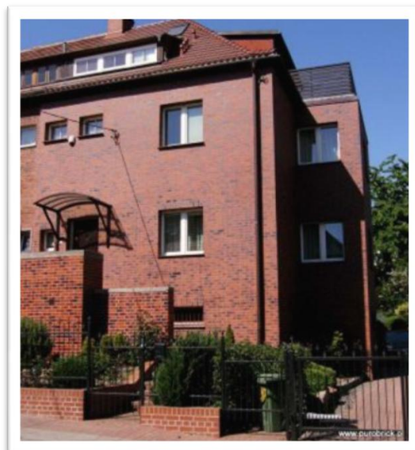
Figure 22 - Building retrofitted with the brick cladding system based on PUR foam (PRE Fasada)
