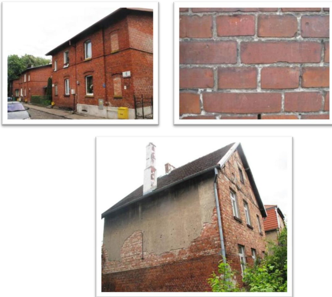
Figure 8 - Example of a residential building constructed from brick without and with plaster
