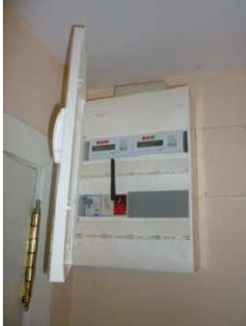
Figure 9: Zaragoza smart meters for partial consumptions monitoring
