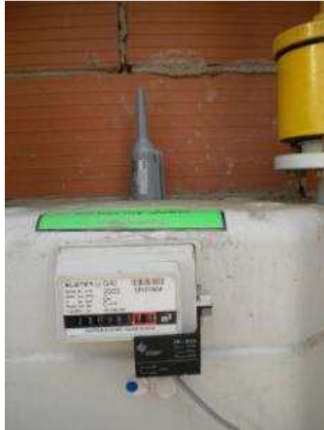
Figure 3: Gas counter from Zaragoza pilot with the telemetry device installed (example of counter that support telemetry)
