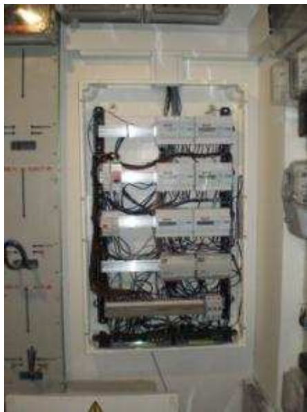
Figure 8: Zaragoza electricity smart meters installed in counters room
