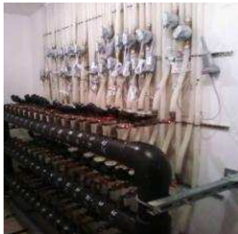
Figure 4: Example of installation of new counters between utility counters and the delivery system in Zaragoza Pilot
