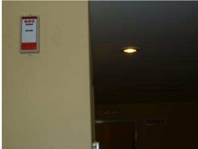
Figure 11: Temperature/Humidity sensor installed in Zaragoza common area
