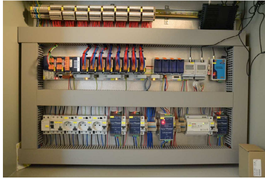
Figure 18: Control cabinet for Warsaw.
