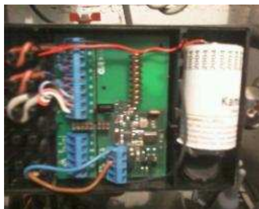
Figure 5: Example of the installation of one accessory in order to make the counter available to support telemetry – Zaragoza pilot
