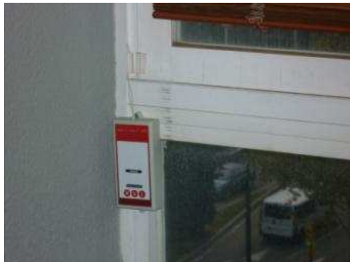
Figure 10: Window sensors installed in Zaragoza
