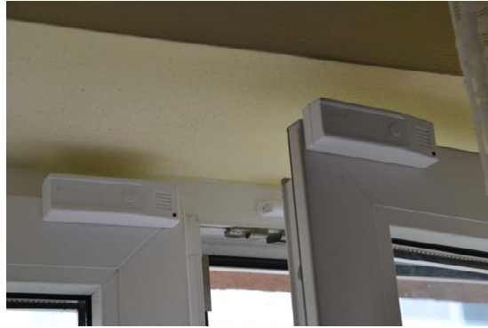
Figure 20: Reed switches for windows (open - close windows sensors).
