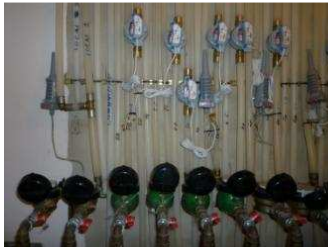
Figure 12: Cold water smart meters in Zaragoza
