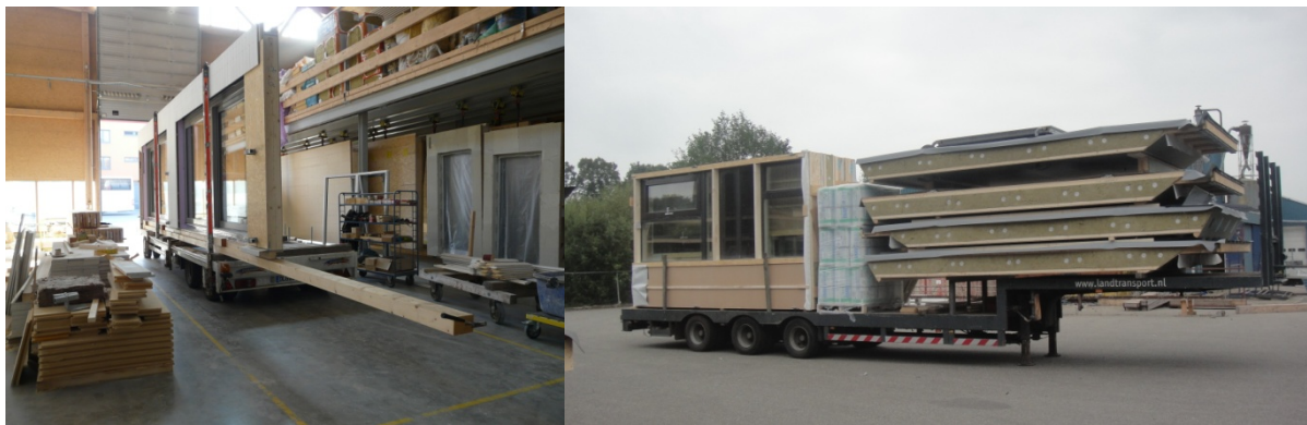
Figure 5 - Loading bay at Gump & Maier . Roosendaal: elements for one house on one truck
