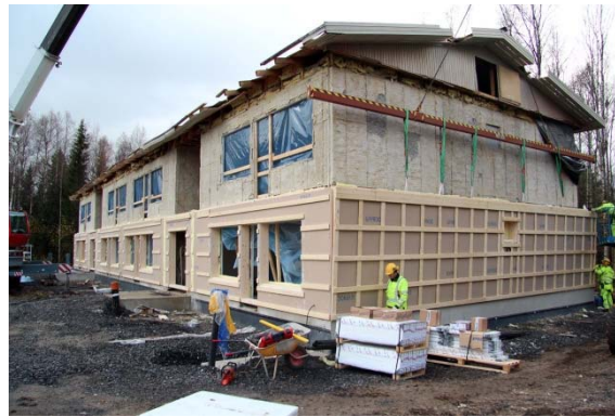
Figure 64: Oulu demonstration during assembly of prefabricated TES elements (Photo: Simon Le Roux).
