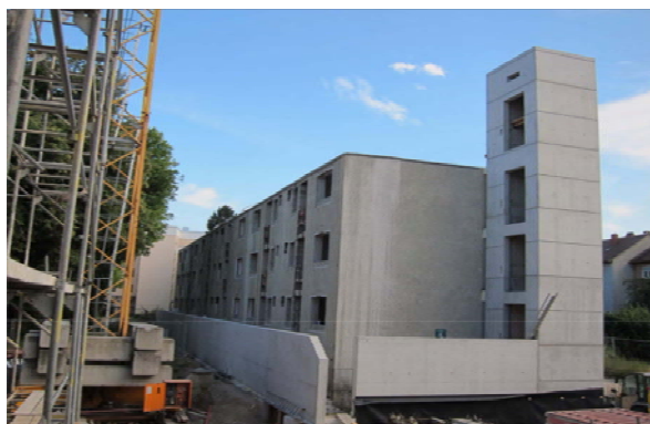
Figure 63: Dismantled structure of Munich demonstration with new elevator shaft (Photo: Lichtblau Architects).
