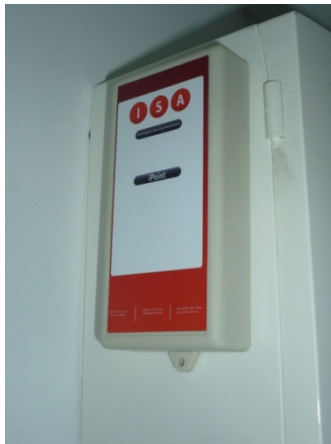
Temperature/humidity sensor installed in a dwelling
