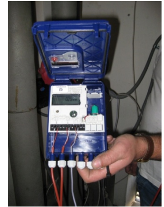
Enthalpy meter used for measuring energy generation through solar panels
