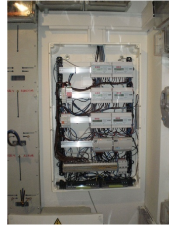
ISA iMeters used for measuring electricity consumption
