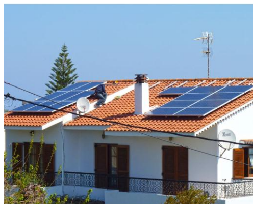
PV panels on the roof of private residence in Rhodes, Greece
